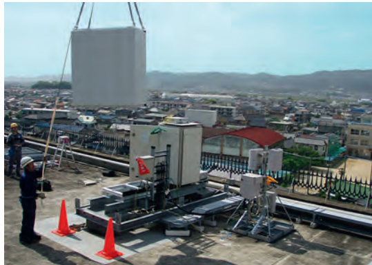
An RBS 3016 is being lifted into its new home as the Ericsson team swaps out the Nokia site.
