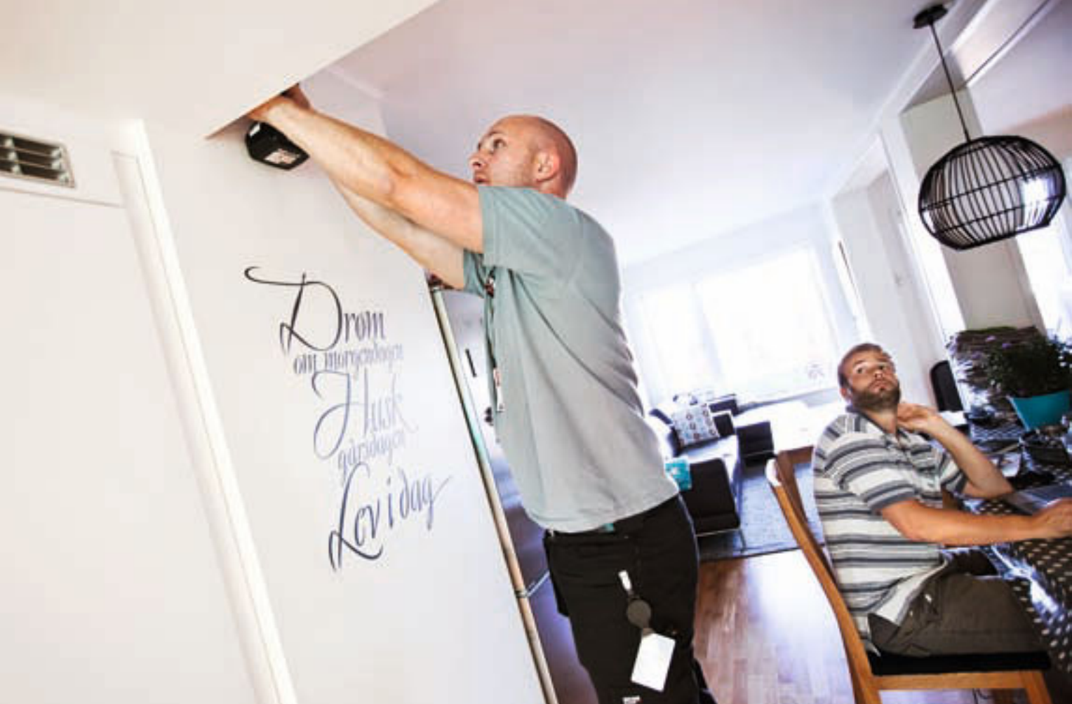
Row-house owner Tony Liavik looks on as John Sundt of Sector Alarm installs a micro camera in his home.
