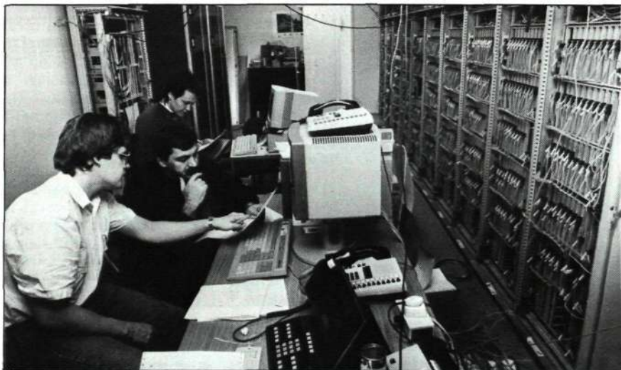
The Easter weekend saw the completion of the toughest phase in installing the world's largest MD 110.
