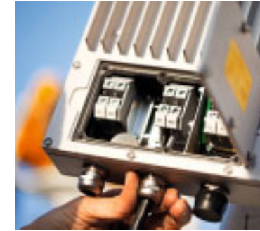
A Remote Radio Unit is installed aboard the Maersk Penang.
