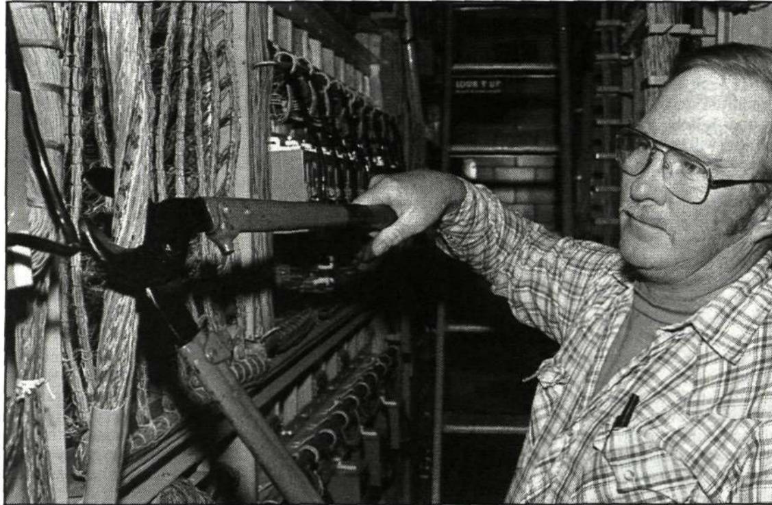
Larry Livingston, a Mountain Bell Cable Splicer, cuts the cables that connected Canon City subscribers to the old step-by-step crossbar switch. The splicing took place seconds before connections were made to the new AXE Digital Switch.
