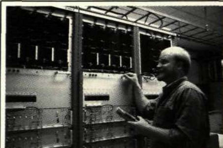
Installation in Pittsburgh of a radio base station for mobile communications.
