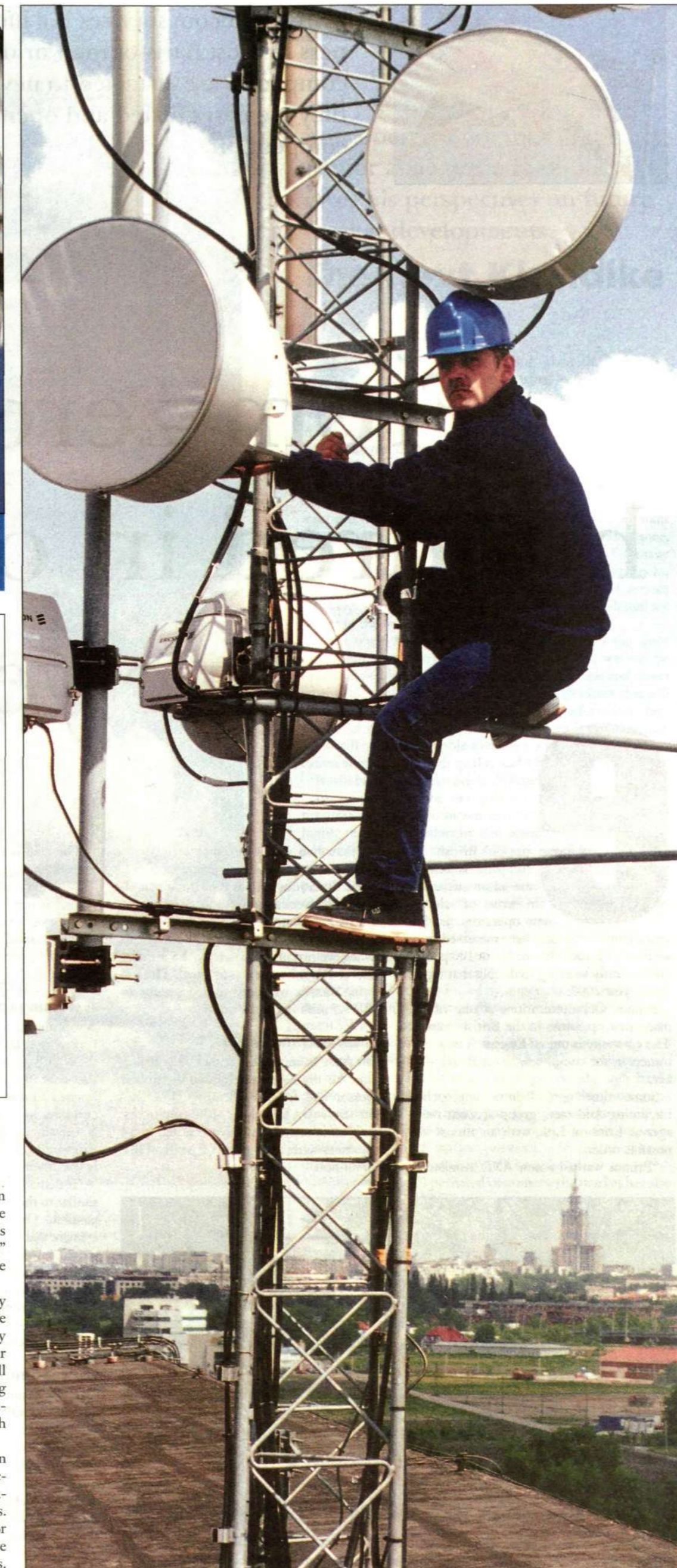
The transmission network is not large enough in Poland, which is why radio links are often used for GSM network expansion. Shown above is Dariusz Drogosiewicz on a tower with a MINI-LINK.
