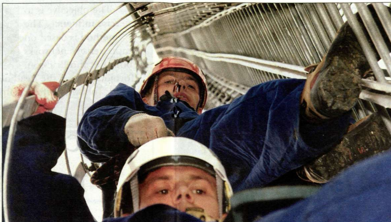
Pawel Pabiniak and Grzegorz Tomczyk are working hard to install radio antennas for the GSM network in Poland.
