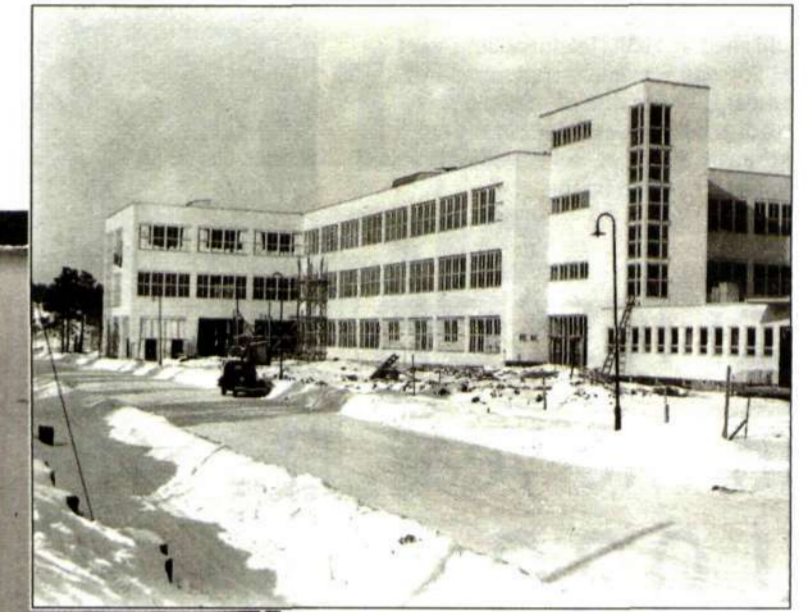
The new main factory (HF) at Midsommarkransen begins to take shape. The picture above shows progress at the construction site on January 19, 1939.
