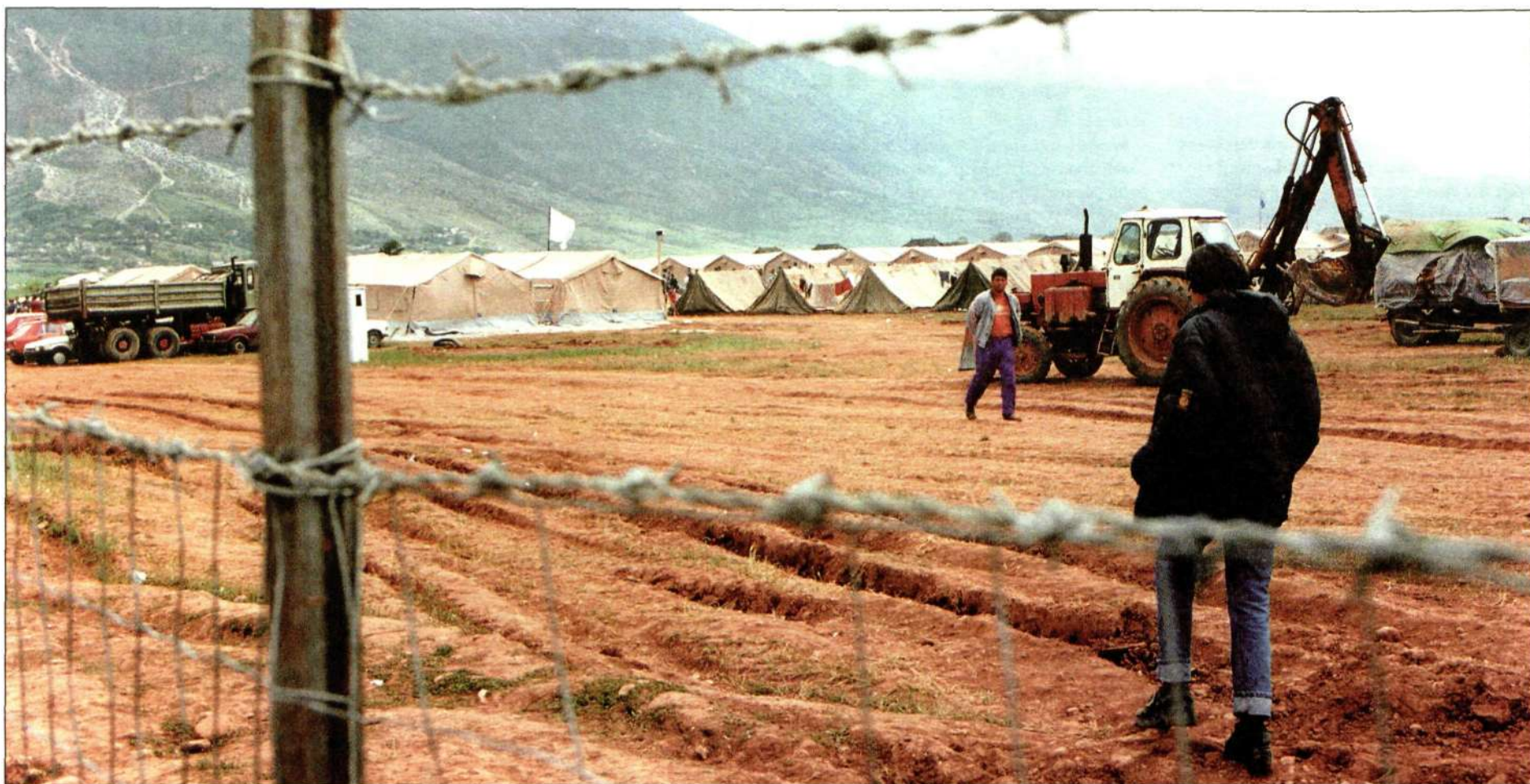
There is an enormous need for telecommunications in Kukes and Ericsson is to construct a mobile network, to help the refugees find their relatives.
