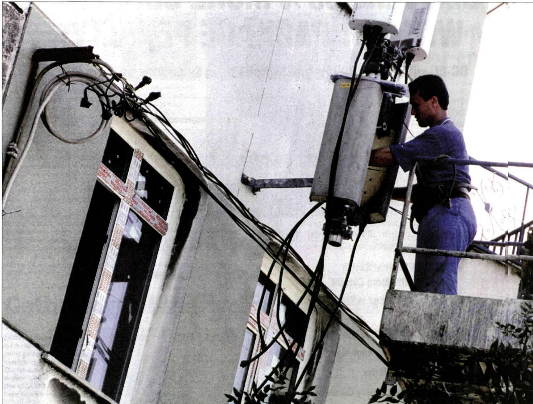
Ericsson is currently carrying out the mass installation of base stations in Turkey as a result of the major order from Turkcell. That is why it was easy to mobilize all resources to quickly restore communications in the affected area. Mehmet Pigak is pictured setting up a base station antenna in the district of Avclar on the outskirts of Istanbul. Photo: Lars Åström
