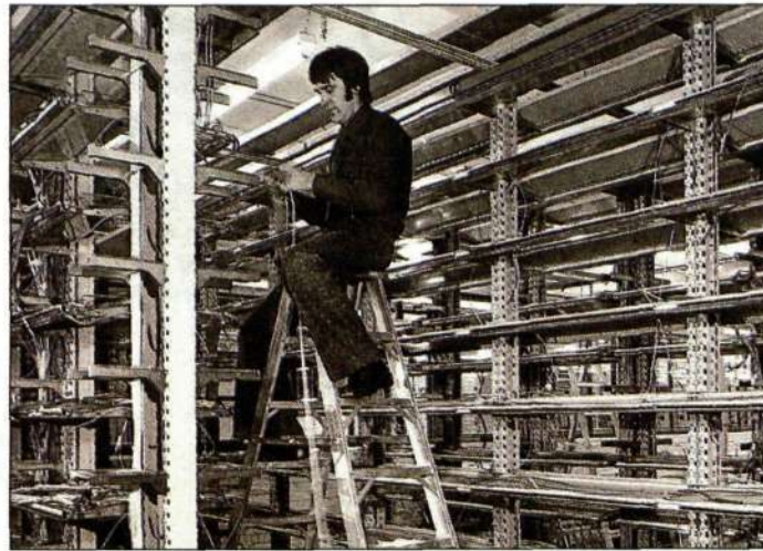
In the 1970s, AXE required an entire building – plus a ladder...
