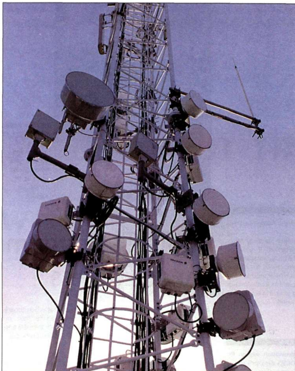
The point-to-multipoint MINI-LINK BAS system is an important part of Ericsson's broadband strategy.
