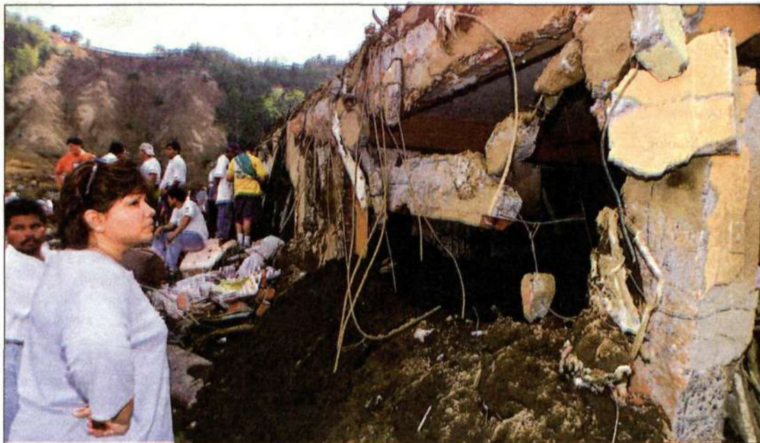
Residents of the La Colina district of Santa Tecla inspect the damage following the recent earthquake. Intensive rescue efforts were in progress, and local Ericsson employees were working overtime to get the mobile telephone network up again.
