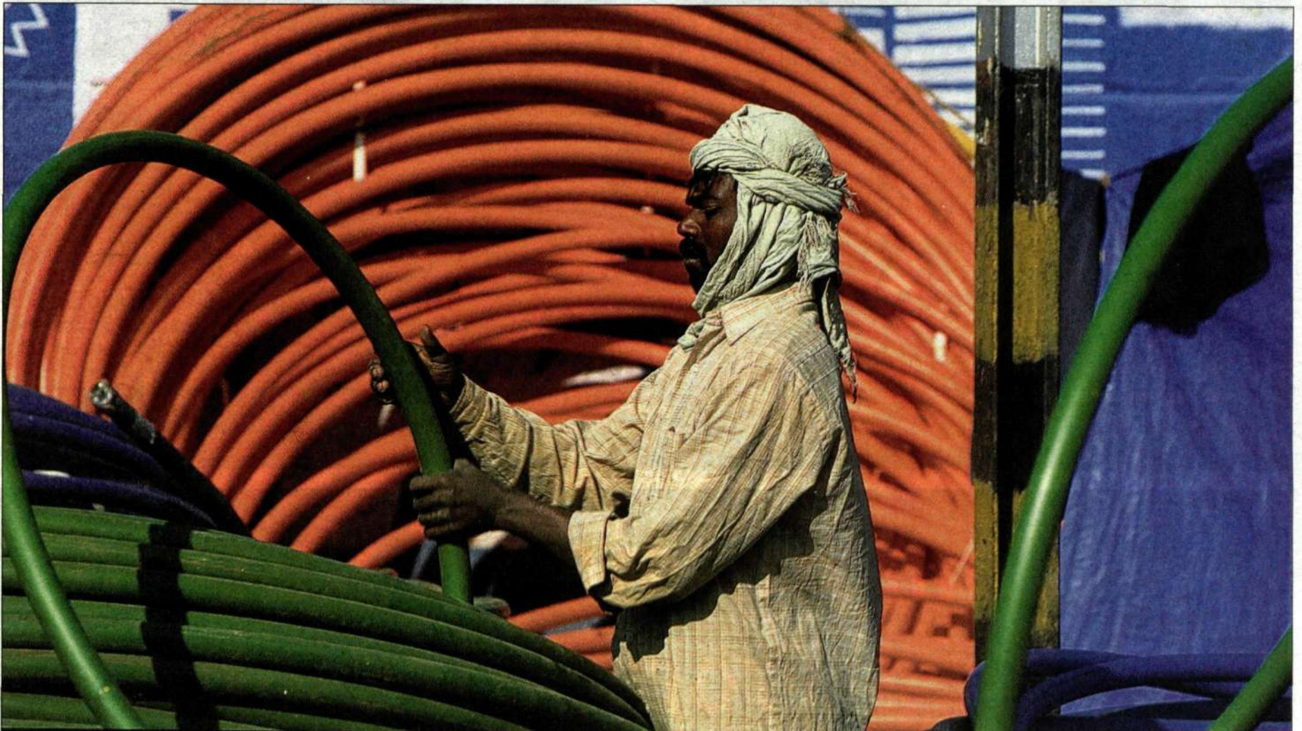
The expansion of broadband fiber-optic networks alongside India's roads is the most visible sign of the country's developing digital infrastructure.
