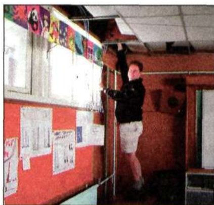
Matt Rowbotham was one of the volunteers at NetDay in Hawke's Bay, New Zealand. He spent one Saturday drilling, feeding and dragging cable through the ceiling of a block of classrooms.
