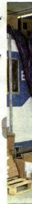
The 3G test system is being installed in three containers; two large ones and one small.
