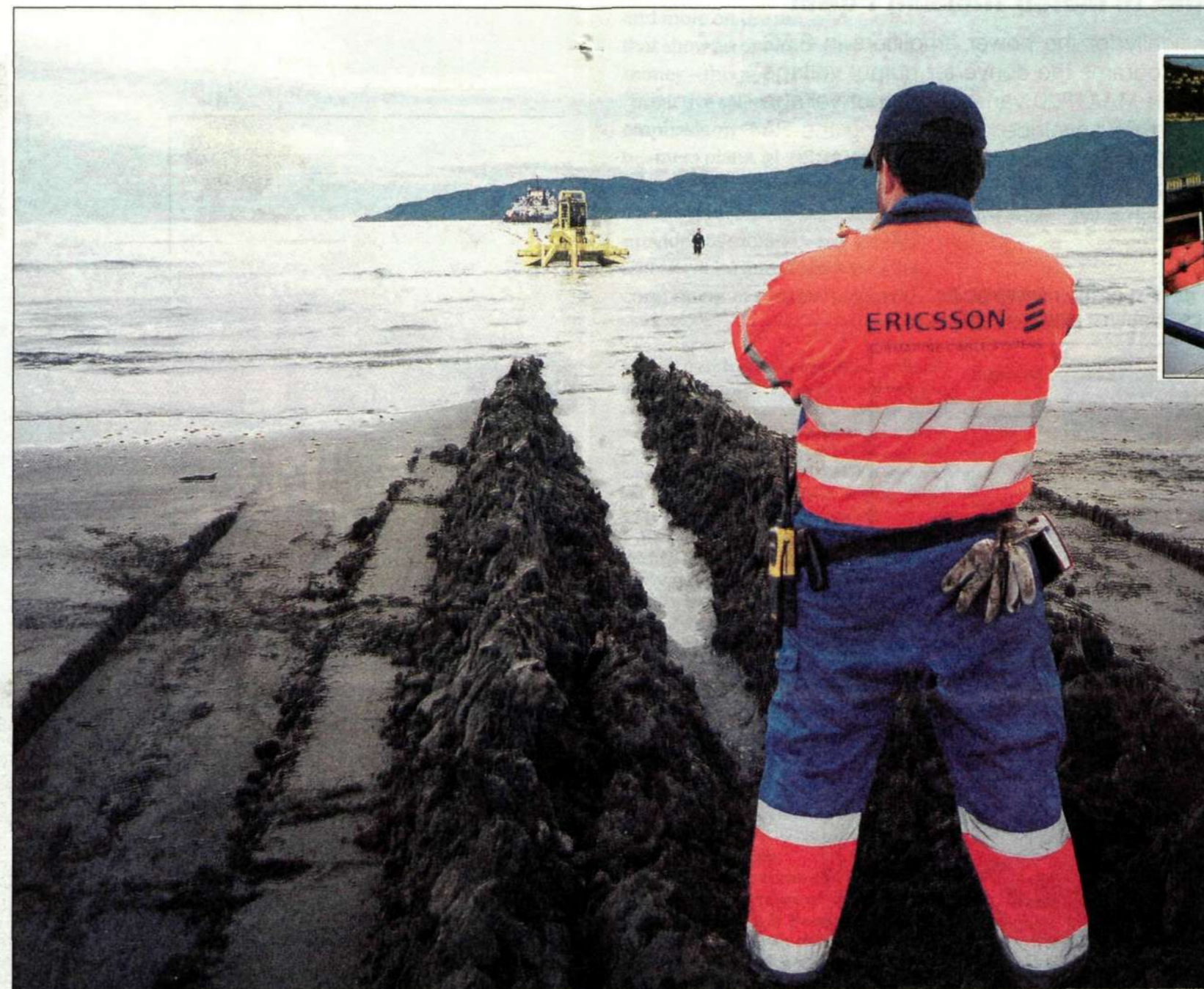
Dan Kenealy, Ericsson's marine specialist, oversees the plough that is used to dig the trench where the cable is laid.
