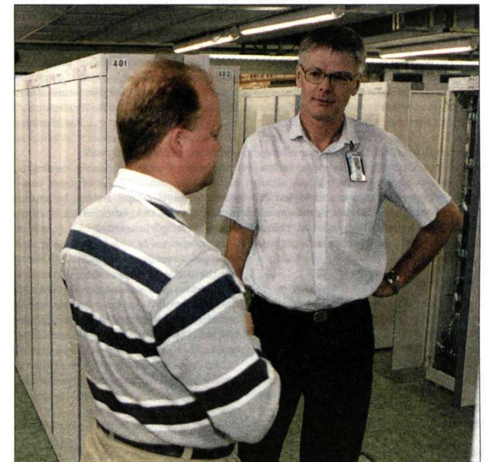
The Linköping test facility has grown strongly and today features mobile switches and BSC units corresponding to two normal-sized telecom networks, according to section manager Mikael Pettersson and general manager of the Design Center, Jack Järkvik.
