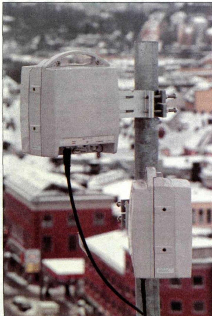
Microwave operations account for about two-thirds of total operations conducted by the new Transmission and Transport business unit, with optical transmission accounting for the remaining one-third. The picture above shows a MINI-LINK BAS microwave installation in Oslo.
