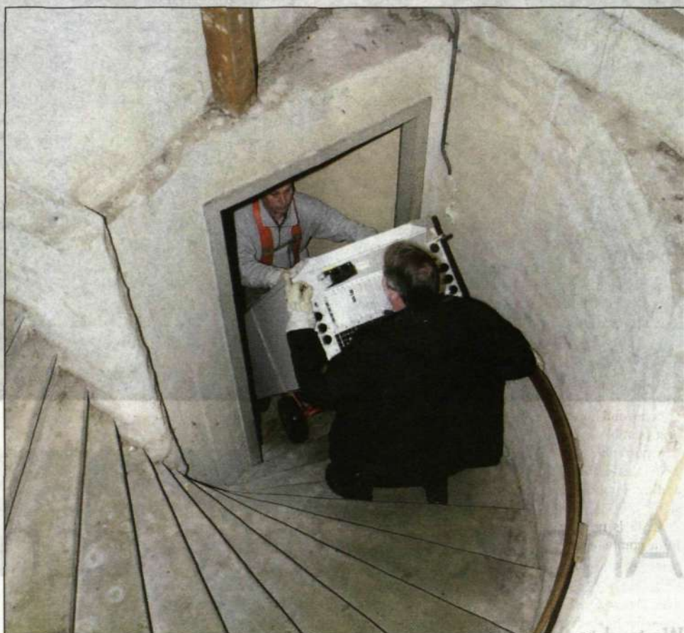
The full-scale rollout of 3G networks is now occurring and operators need plenty of assistance. Ericsson has the ability to provide customized support. Here, a WCDMA base station is being installed in Sweden.
