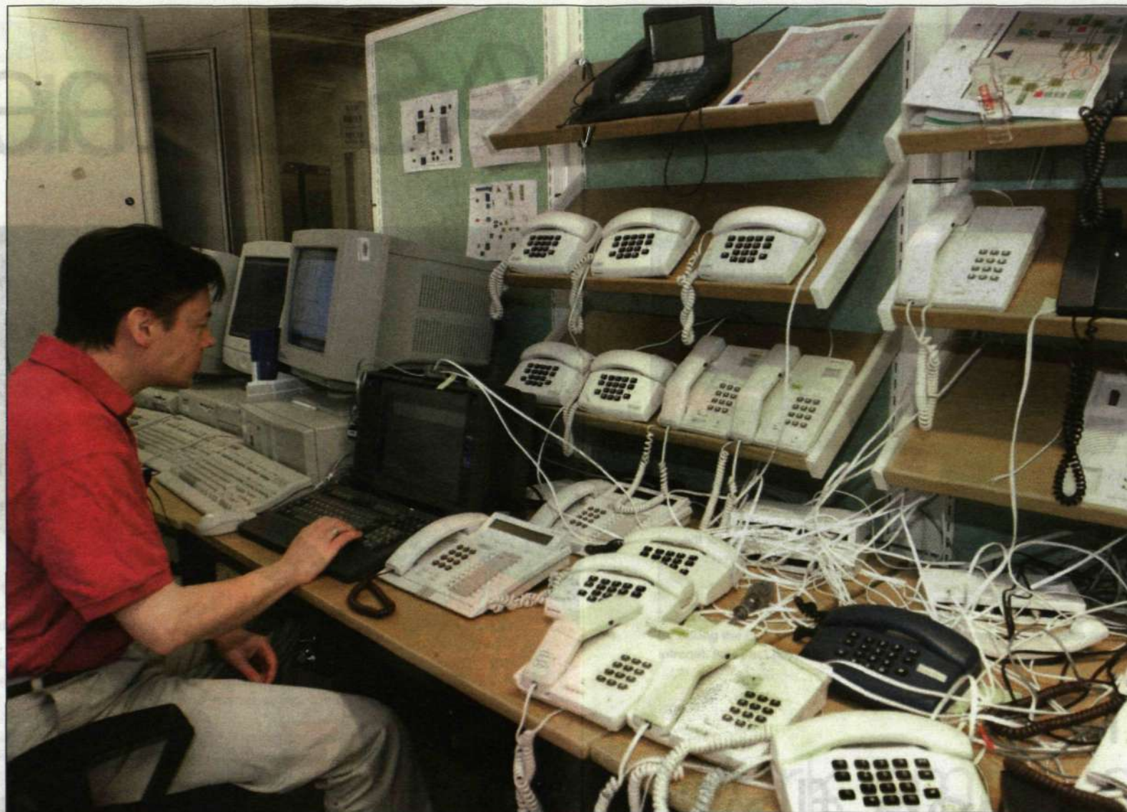
A large number of the AXE switches manufactured are used by Ericsson for testing. Most systems and solutions are adapted according to customer requirements and are carefully tested and verified prior to delivery.
