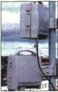
MINI-LINK BAS installation.
