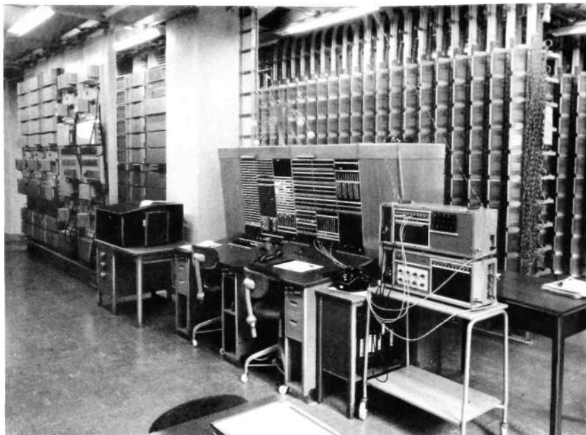
Fig. 10 X 8182 Traffic supervisor's desk and equipment for traffic metering
