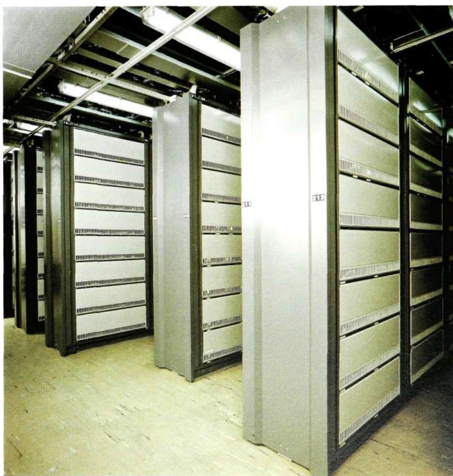
Fig. 2 The 10 000-line AXE local exchange at Al Ulaya
