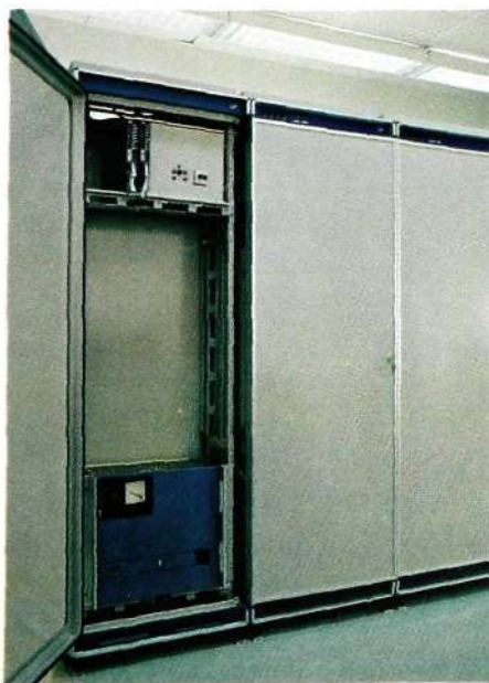
Fig. 8 Rectifier BMT 243 (25 A) in PABX ASB 900. A distribution unit (BMG 660001), which is specially adapted for this PABX, is mounted at the top of the rack. The distribution unit contains automatic fuses, a printed board assembly for supervision of the distribution voltage and automatic charging and a special alarm collecting board
