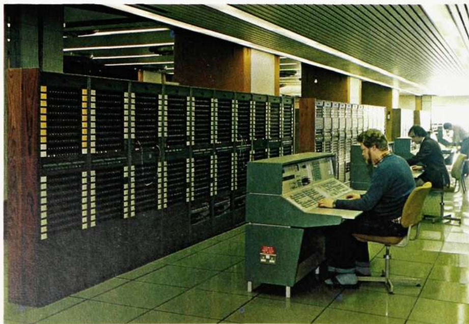
Fig. 7 The International Transmission Maintenance Centre in London/Thames ISC with signalling links for signalling system No. 6 on the left
