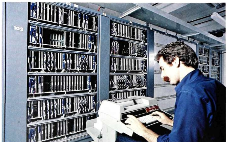
Fig. 10 Exchange equipment and maintenance terminal
