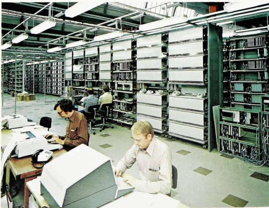
Fig. 6 Pre-test plant for overall testing of complete exchanges before delivery
