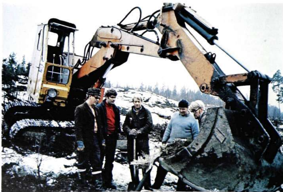
Fig. 1 Accidents will happen — an excavator has damaged a telecommunications cable
