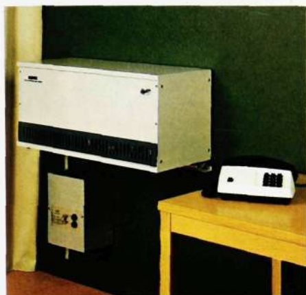
Fig. 8 The central equipment can be placed in an ordinary office environment
