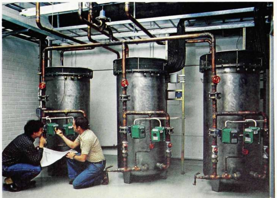
Fig. 5 Water-cooled load units are placed in stainless steel tanks. The left tank is used for AC loads. Maximum load 200 kW. The other two tanks, which are used for DC loads can together be loaded with 7500 A at 50 V (375 kW)
