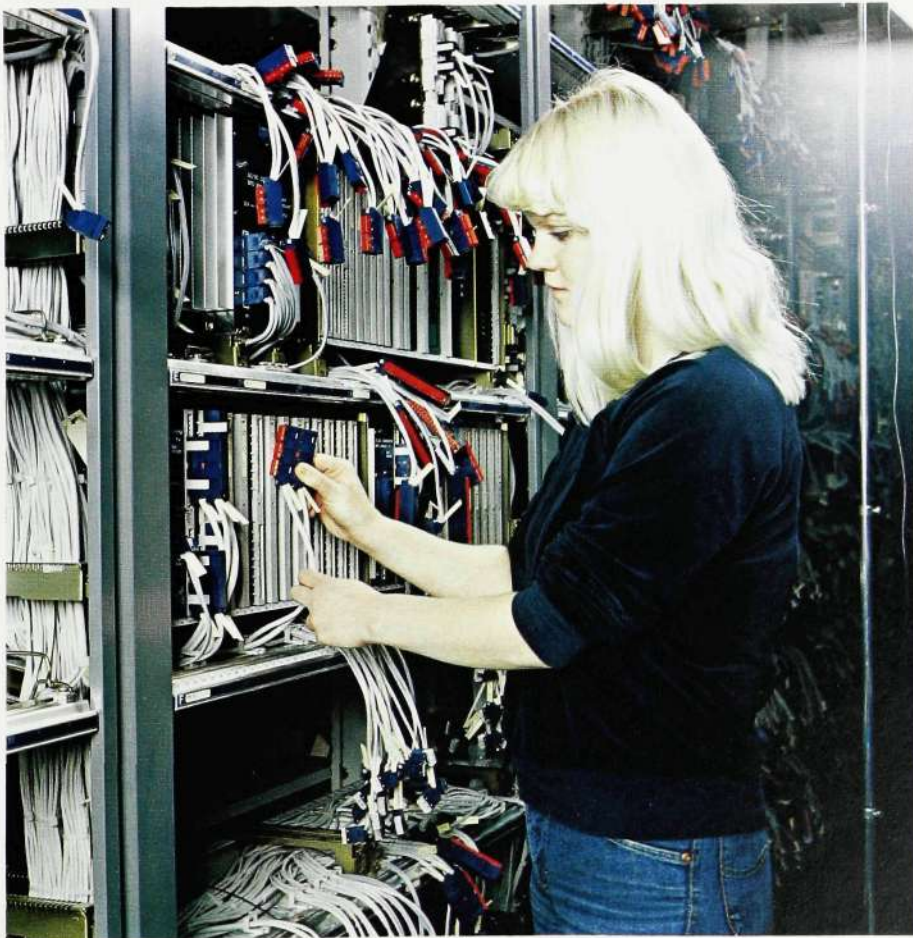
Fig. 8 Cables are plugged into jacks and terminals strips
