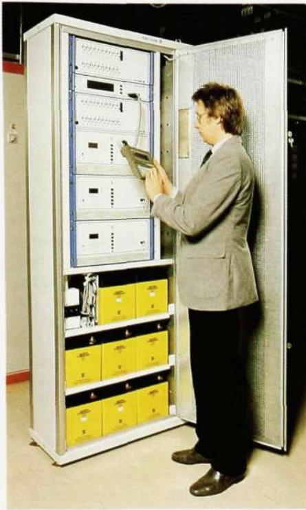
Fig 5 BZA 204 03/13 This system differs from BZA 204 05 in that the battery is placed in the same cabinet as the rectifiers and distribution units
