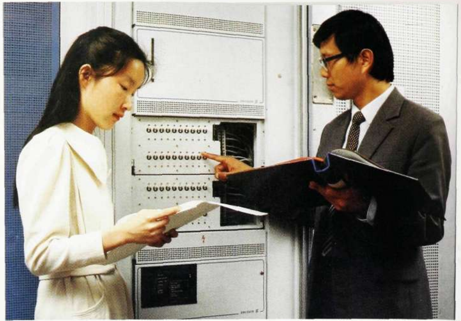
Fig 9 Great interest has been shown in the new power supply equipment. Presumptive customers study the equipment at Telecom 87 in Geneva
