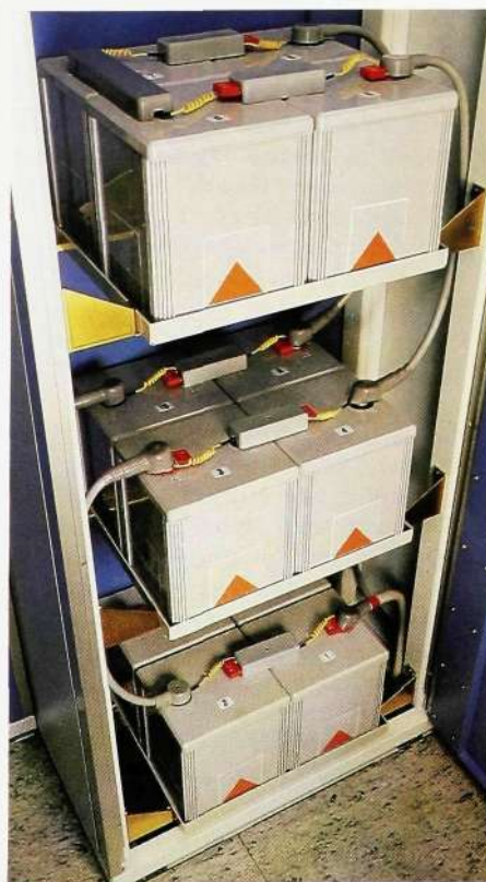
Fig 6 Sealed battery with cell voltage equalizers, installed in a BYB cabinet
