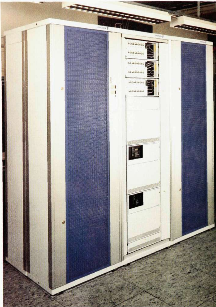
Fig 4 BZA 204 05 New power supply equipment with 50 A rectifiers, designed for installation together with AXE 10. The door of one of the power cabinets has been removed. The rear row contains a battery cabinet
