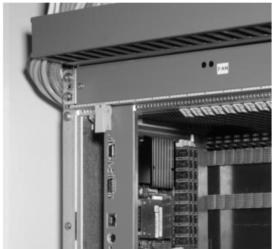
Figure 2 Typical hardware subrack for Ronja.
